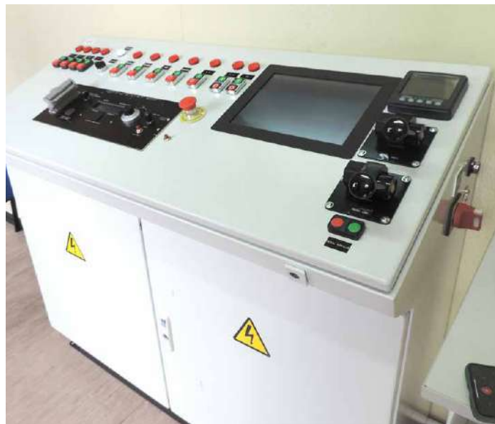
> The entire inspection procedure is managed from the control room, where DEUTZ also runs training courses for technicians.
